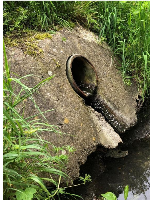
Photo 4-28: SD2 module 1 outfall
